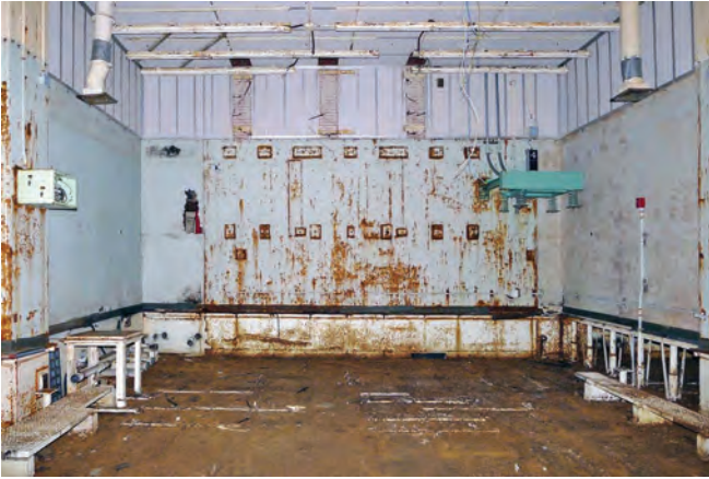
Contemporary photo of the stripped BMDOC. The raised floor and suspended ceiling have been removed
